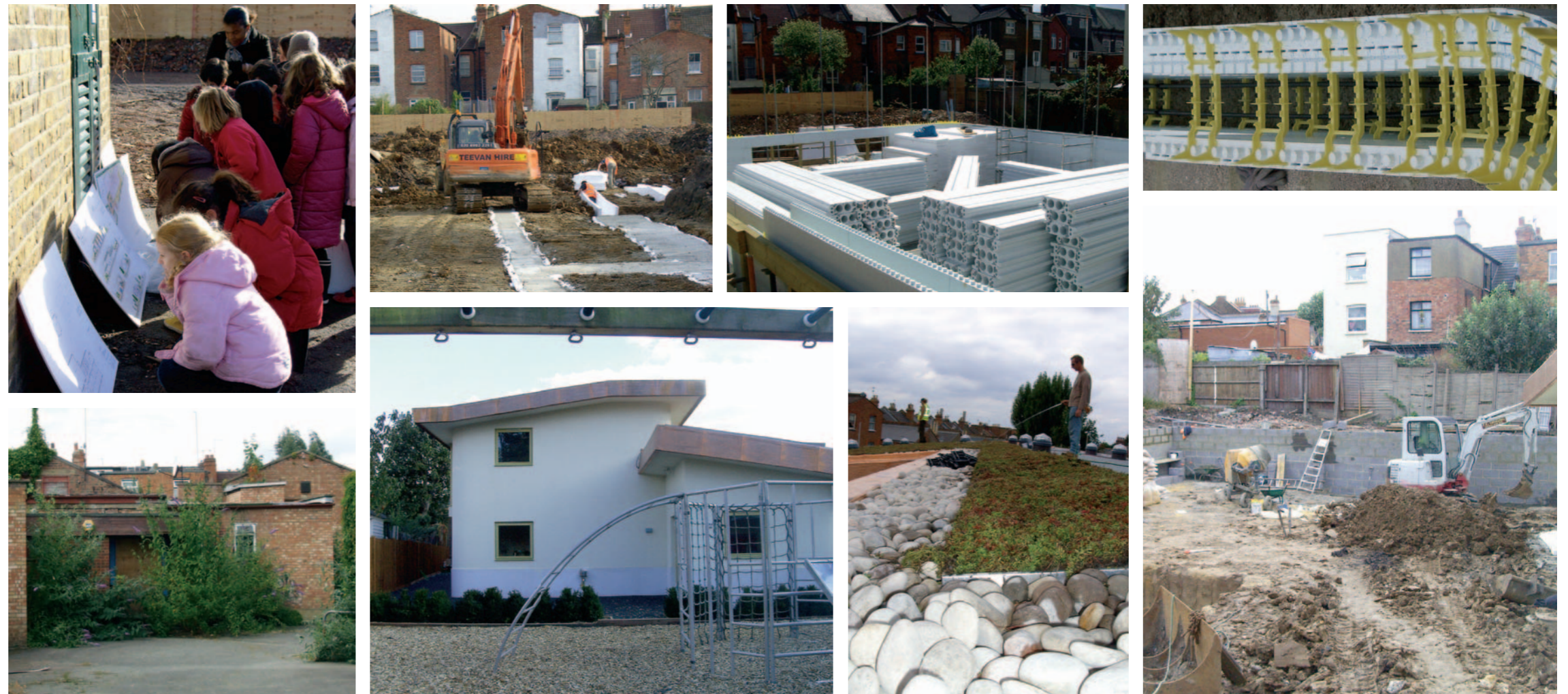
Pictures (Clockwise from bottom left): The old social club before demolition, Maple Walk pupils inspect plans after demolition, foundations are laid, Quad-lock casings are constructed, the Quad-Lock system in detail, the site overlooked by the local neighbourhood, the sedum roof is watered, the build is finished.
